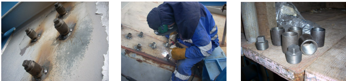
Pictures showing installation of coupling and caps and a field of seam connector pattern
